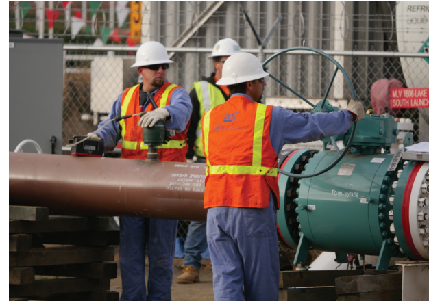
SDG&E has upgraded more than 23 miles of transmission pipeline in San Diego County as part of our Pipeline Safety Enhancement Plan.
